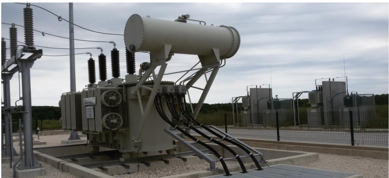
Slika 2.1: Energetski transformator, TS Funtana
